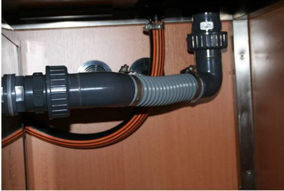
Fig. 2: Drainage fittings installed. The striped pipe behind is the flexible hose that connects the Eco Runner 3700 to the hosetail on the bottom of the 25 mm rigid pipework tank connector.
